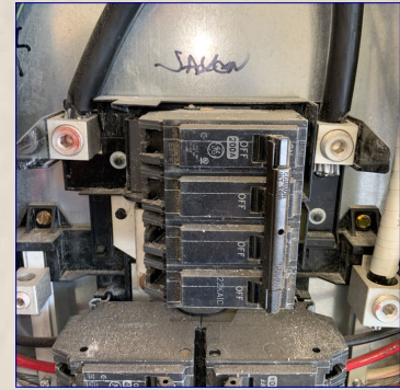
The main electrical service panel shut off breaker.
