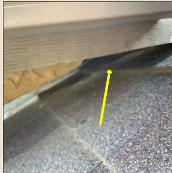
There were areas of missing flashing. Recommend a licensed roofer install flashing.
