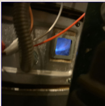
The water heater operating.
