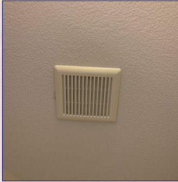
The exhaust fan operating.
