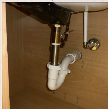
The bathroom plumbing view.
