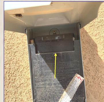
The air conditioner compressor/condenser electrical shut off switch.
