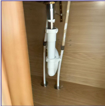
The bathroom plumbing view.
