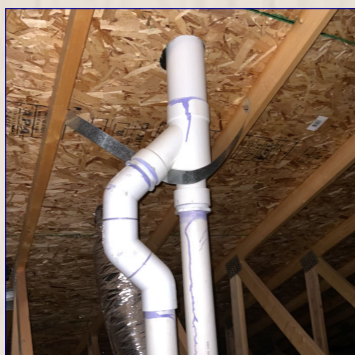
Hvac plumbing view
