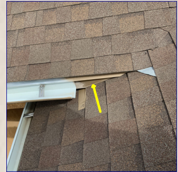
The fascia needs routine painting maintenance. Recommend a professional painter repair/paint the fascia.
