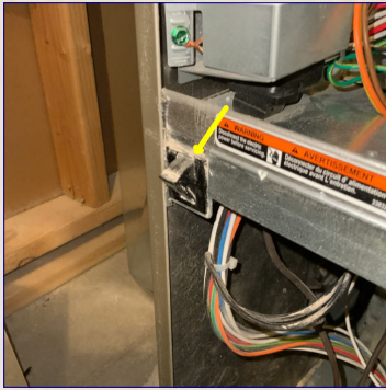
The electrical shutoff switch.
