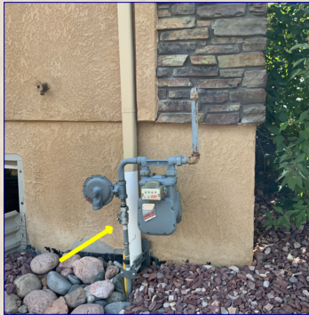
The main gas shutoff valve.
