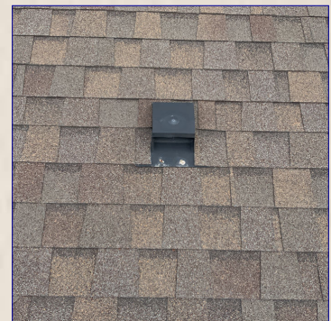
The Bathroom Vent(s)
