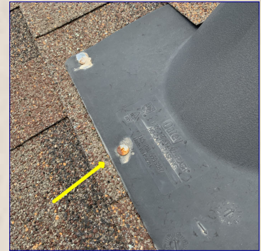
There are exposed nail heads securing the flashing to the roof. Exposed nail heads can allow water to penetrate the roof. Recommend a licensed roofer to seal the nail heads.
