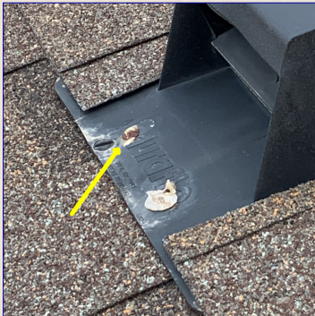
There are exposed nail heads securing the flashing to the roof. Exposed nail heads can allow water to penetrate the roof. Recommend a licensed roofer to seal the nail heads.
