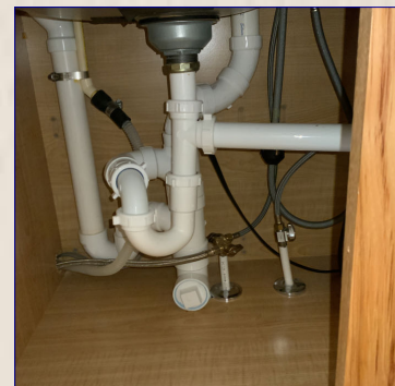
Kitchen plumbing view
