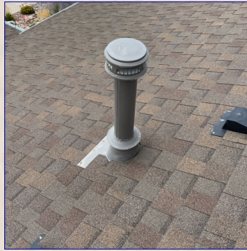
The HVAC Vent(s)
