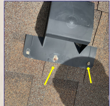
There are exposed nail heads securing the flashing to the roof. Exposed nail heads can allow water to penetrate the roof. Recommend a licensed roofer to seal the nail heads.
