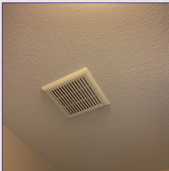
The exhaust fan operating.
