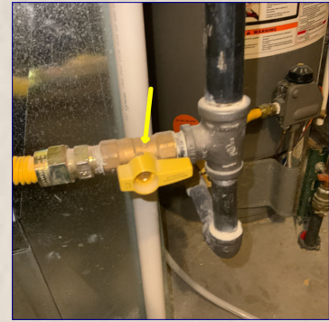
The gas shutoff valve.
