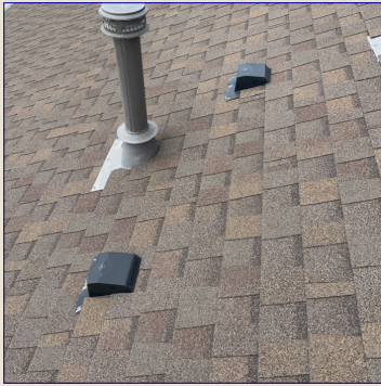
The Bathroom Vent(s)
