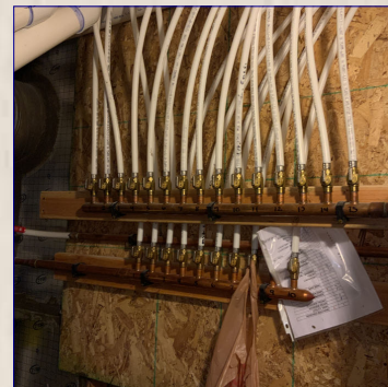
The main water diaphragm shutoff system.
