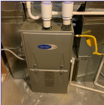
The furnace area
