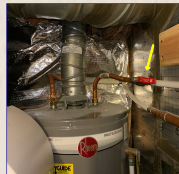
The Water Heater water shut off valve.
