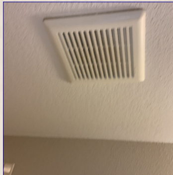
The exhaust fan operating.
