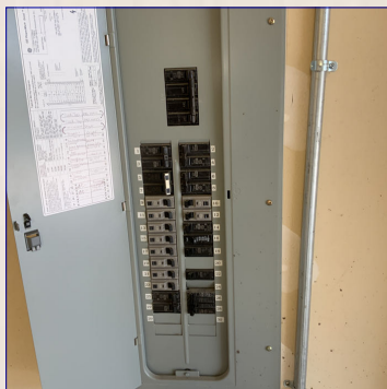
The main electrical service panel.
