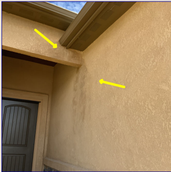
The stucco had moisture staining. Recommend a licensed contractor evaluate and repair as needed.
