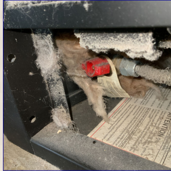
The fireplace gas shut off valve.
