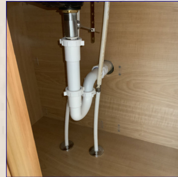
The bathroom plumbing view.
