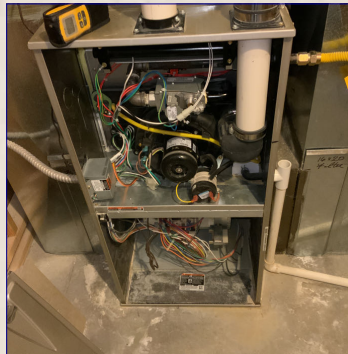
The furnace view, cover off
