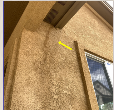
The stucco siding had moisture staining. Recommend a licensed contractor evaluate and repair as needed.
