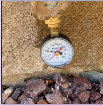
The water pressure at the hose bib.
