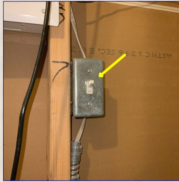
The electrical shutoff switch.
