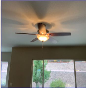
Ceiling fan operating
