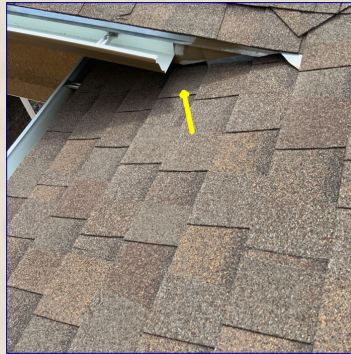
The fascia needs routine painting maintenance. Recommend a professional painter repair/paint the fascia.
