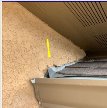
Kick Out flashing is missing at one or more locations, which may allow moisture damage on the home's exterior, walkways, and driveways. Recommend a licensed contractor install flashing to help properly move water to the gutter system. Repair damaged areas as needed.
