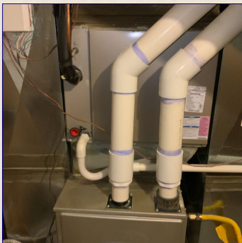
The evaporator coil cabinet.
