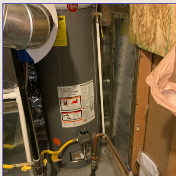
The Water Heater Area
