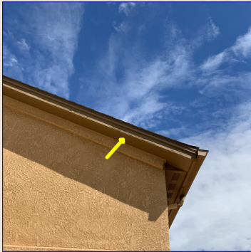
The fascia needs routine painting maintenance. Recommend a professional painter repair/paint the fascia.
