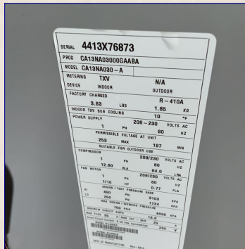
The air conditioner compressor/condenser data plate.
