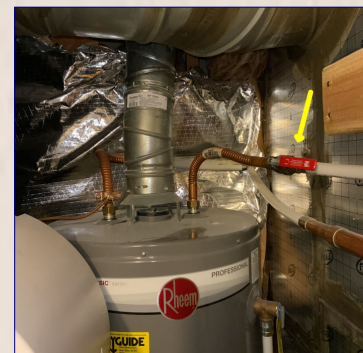
The Water Heater water shut off valve.
