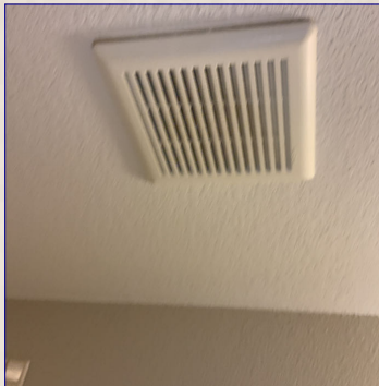
The exhaust fan operating.
