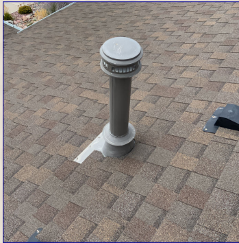
The HVAC Vent(s)
