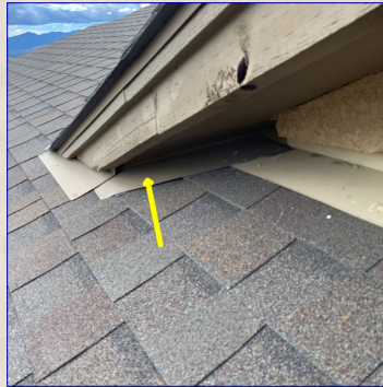
There were gaps at the flashing. Recommend a licensed roofer evaluate repair as needed.
