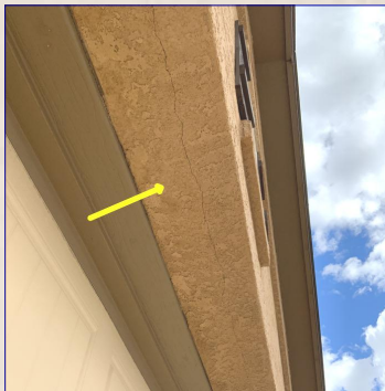
The stucco siding had typical cracking present in one or more areas. Monitor and repair as needed.
