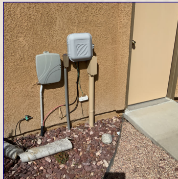
The electrical service entrance.
