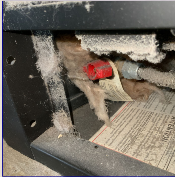
The fireplace gas shut off valve.
