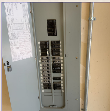
The main electrical service panel.
