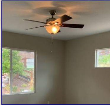
Ceiling fan operating
