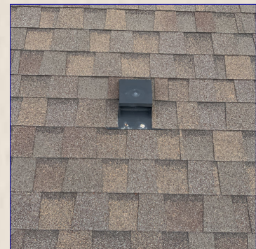
The Bathroom Vent(s)
