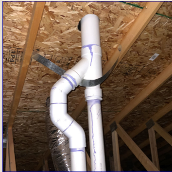
Hvac plumbing view
