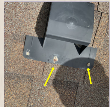
There are exposed nail heads securing the flashing to the roof. Exposed nail heads can allow water to penetrate the roof. Recommend a licensed roofer to seal the nail heads.
