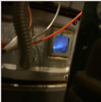
The water heater operating.
