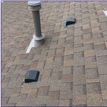
The Bathroom Vent(s)
