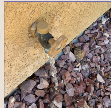
Hose bib operational.
