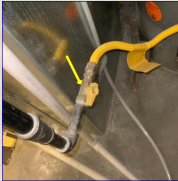
The Water Heater gas shut off valve.
