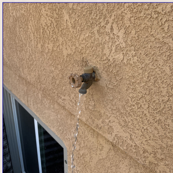
Hose bib operational.
