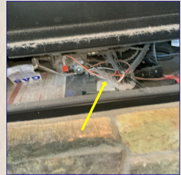
The fireplace compartment was dirty. Recommend cleaning compartment.
