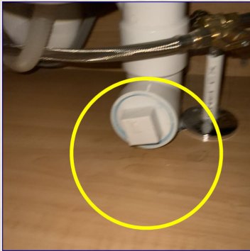
Drains in the kitchen are leaking, recommend a licensed plumber repair.
