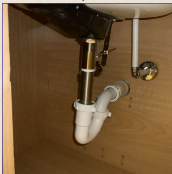
The bathroom plumbing view.
