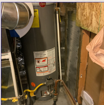
The Water Heater Area
