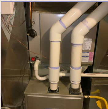
The evaporator coil cabinet.
