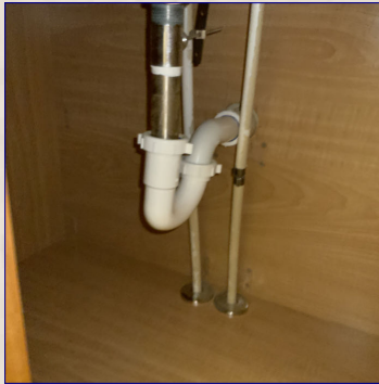
The bathroom plumbing view.
