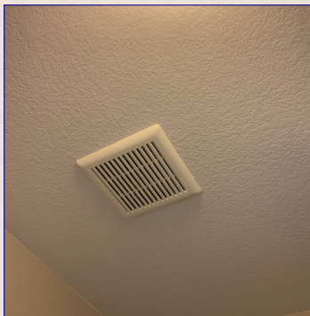
The exhaust fan operating.
