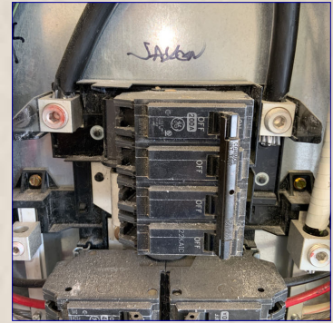
The main electrical service panel shut off breaker.
