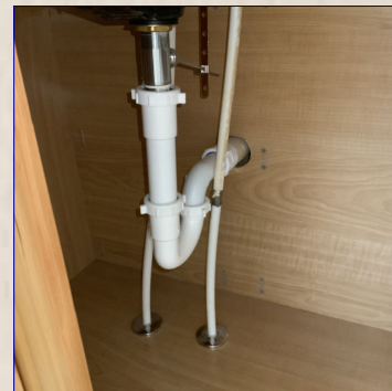
The bathroom plumbing view.
